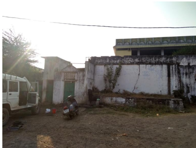
Figure 4.7 Encroachments around the Masjid make it inaccessible
