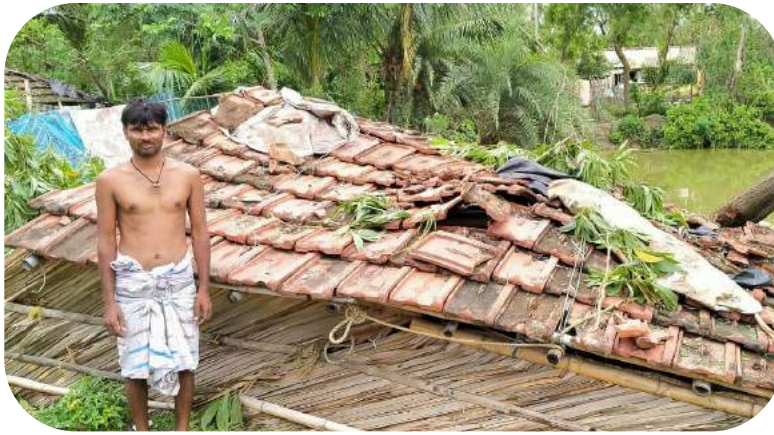
Figure 81 Collapsed Kuccha House (Source: Photo obtained from village over electronic source)
