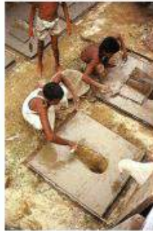
PIT LATRINE UNITS
