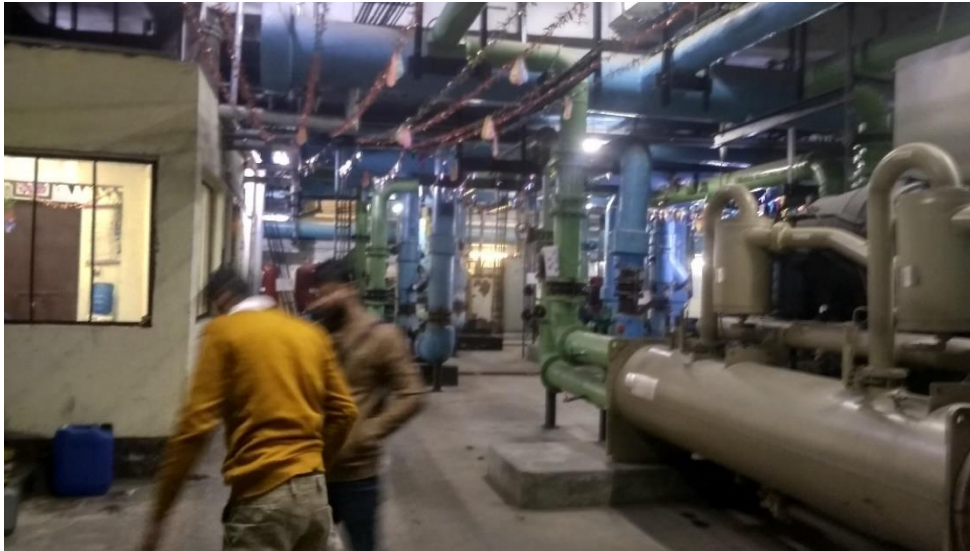
Fig. 7.1.13 HVAC [Image Source: Author]
