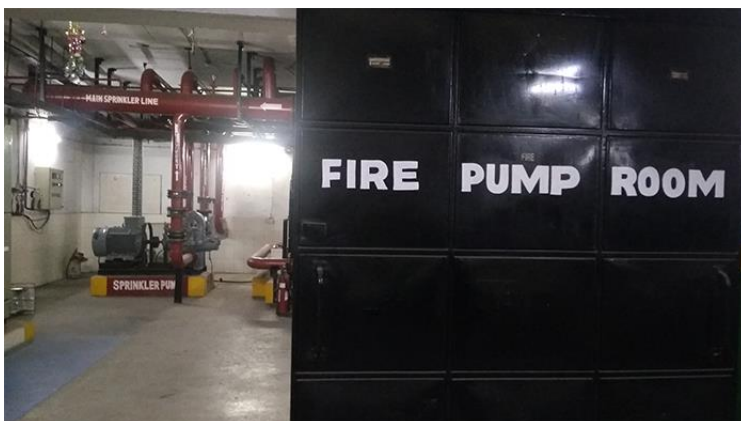
Fig. 7.1.16 Fire Pump Room [Image Source: Author]
