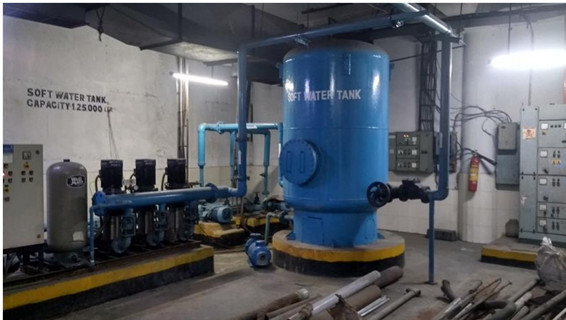
Fig. 7.1.15 Water Supply Room [Image Source: Author]
