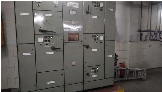
Fig. 7.1.14 Substation [Image Source: Author]
