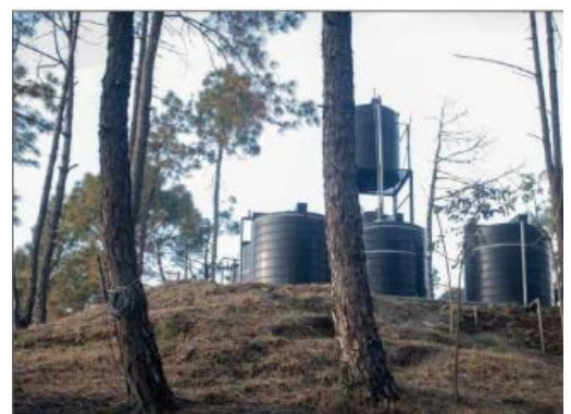
Figure The water from these tankers is pumped to storage tanks and the highest contour level of the site and is then distributed throughout the site through pipes.
