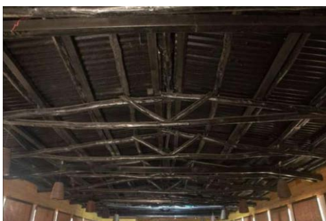
Figure Wooden truss for roof and further supported by steel sections in conference room
