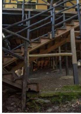
Figure The structures are made on stilts which are wooden but also have steel C sections.
