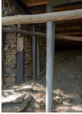
Figure Supporting members provide additional strength to the structure and prevent any mishaps incase a rotten wooden member needs to
