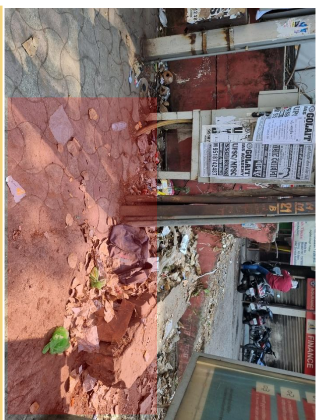
Abrupt end on the sidewalks.
