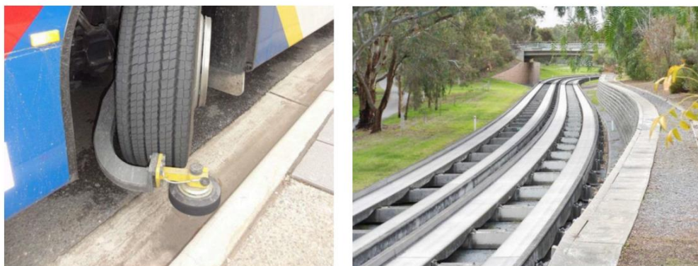
Figure 9 Image showing kerb-guided technology and Infrastructure
