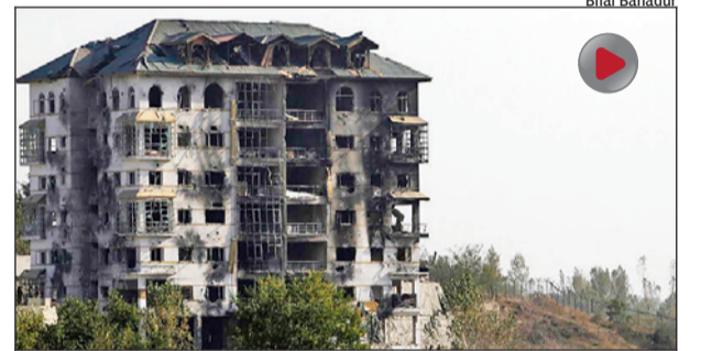
The building where two militants had taken refuge during the gunbattle in Pamore. The 60-hour encounter ended on Wednesday
