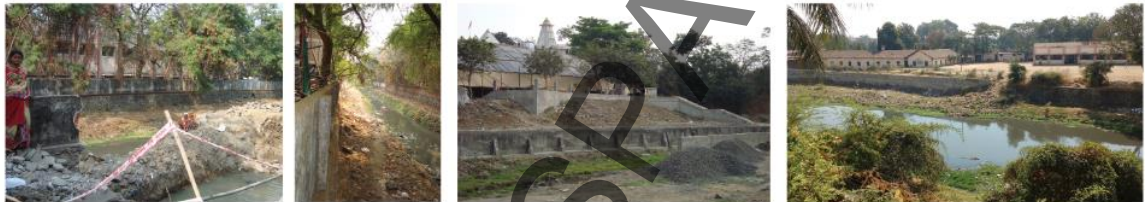
Fig 4.18 Poor Edge along the River Nag (Source: Author's site observations)
