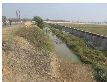
2 Front- adjacent NH2B, Drain
