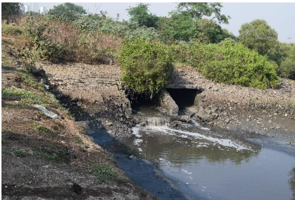
Figure 55 City sewer outlet to the Mangrove
