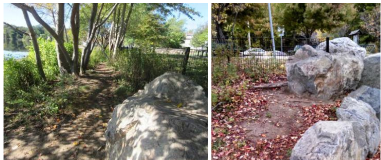
Figure 29: Foot Paths in Plant Beds with Compacted Soil and Erosion.
