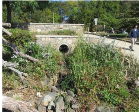
Figure 32: Storm Water Outflow
