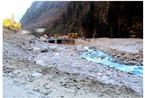
Fig.2.14. Dam destroyed in Vishnuprayag SOURCE: (Circleofblue, 2014)
