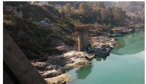
Exposed bedrock turns the river in other direction ,generally low density settlements are present in these areas
