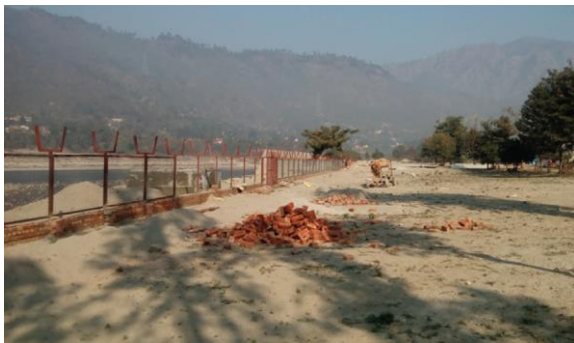
H. Sedimentation yield was highest in this portion, created meters of silt deposition in this area. Retaining wall of concrete has been constructed sometimes ranging up to 7 m from base level.
