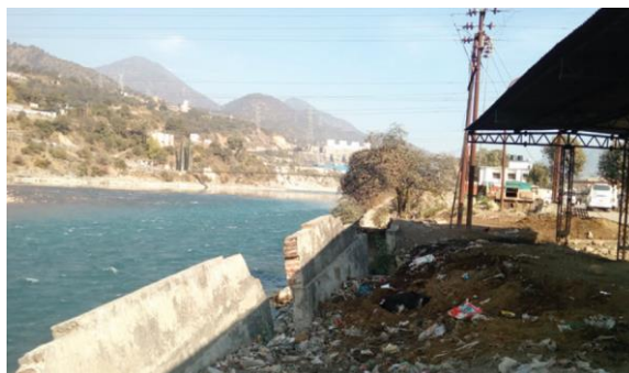
D. Concrete retaining wall creates ecological problems between water and land. In a long run it is failure as dead load increases with base flow. Important public transport route goes in this zone with one bus stand.
