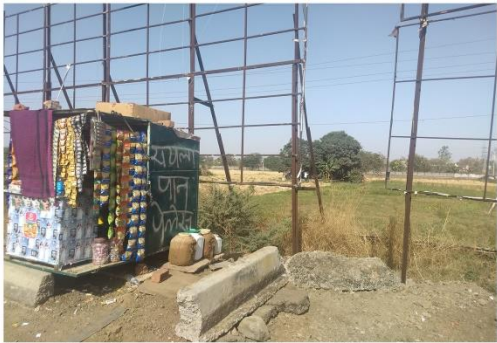
Illegal hawkers, dilapidated condition of edges
