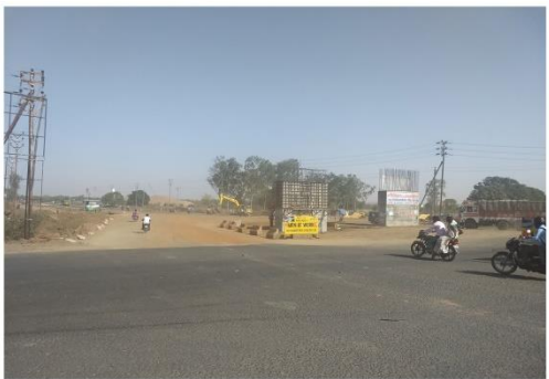
Incomplete flyover, dust and noise
