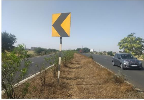
Absence of vegetation on median and lack of signages
