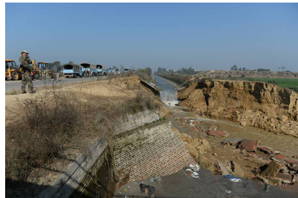
Figure 14: Damage Portion of Munak Canal
